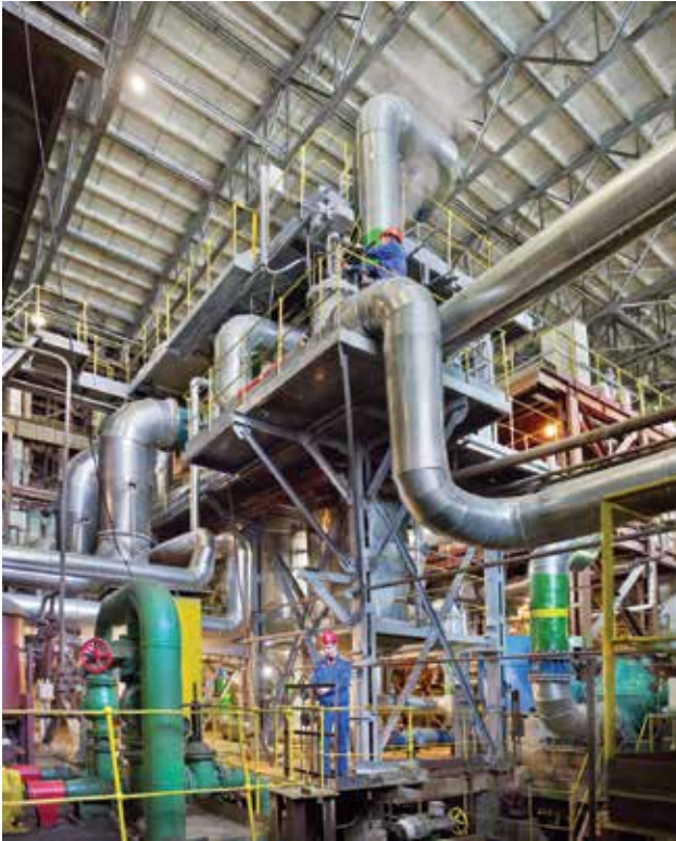
New delivery water pre-heating plant for Ryazan heating supply
