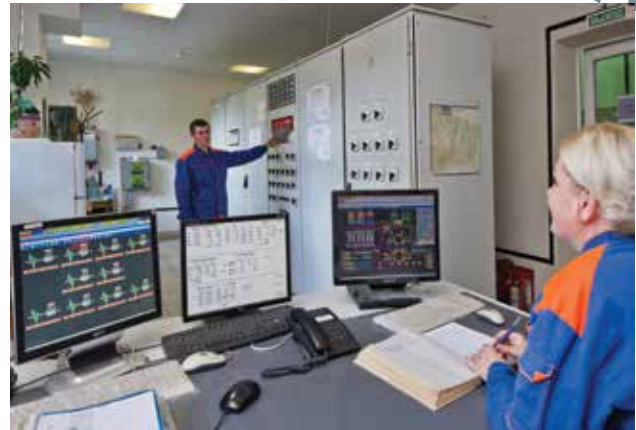
New fuel oil facility's switchboard
