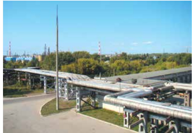
CHP Plant's mains for heating supply of industrial consumers
