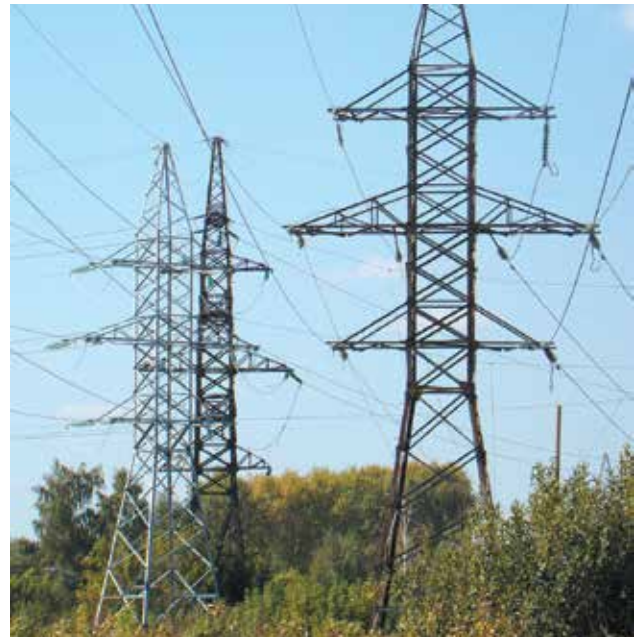
Power lines from CHP Plant to industrial consumers
