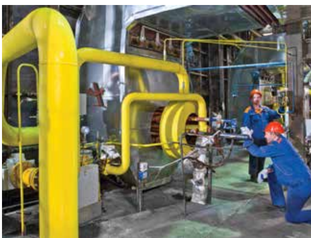
Equipment of new gas facility of Boiler Unit #6
