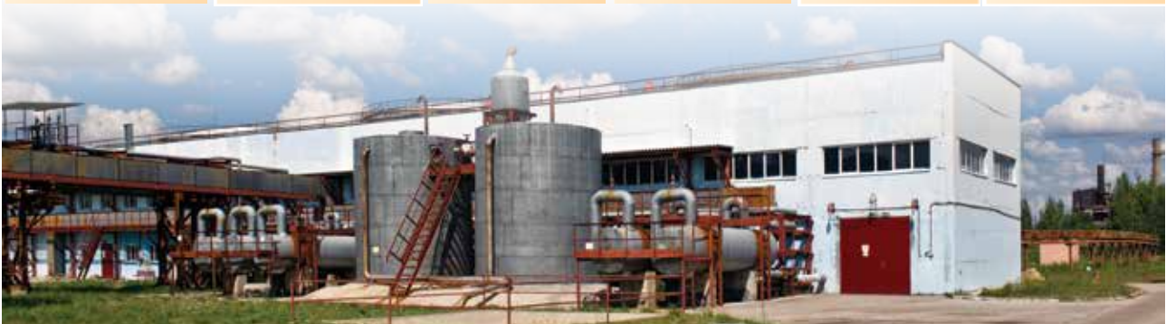
Boiler Department. Pump station of fuel oil facility
