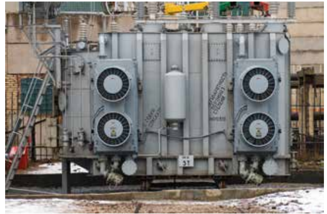
New Power Transformer #5T
