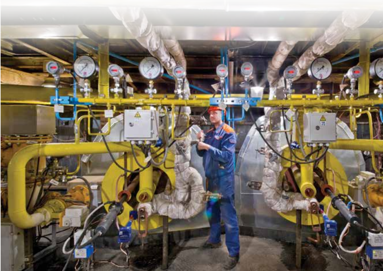
New double flow gas burners on Boiler Unit #6 after upgrading its gas facility
