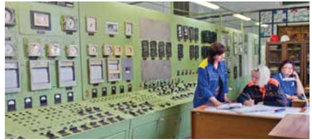
Control board of Chemistry Department's shift supervisor (CWT-1)
