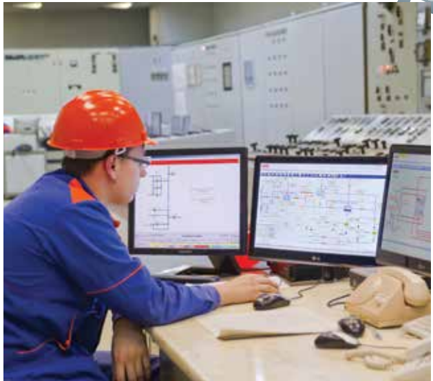
On the control switchboard of the delivery water pre-heating plant for Ryazan
