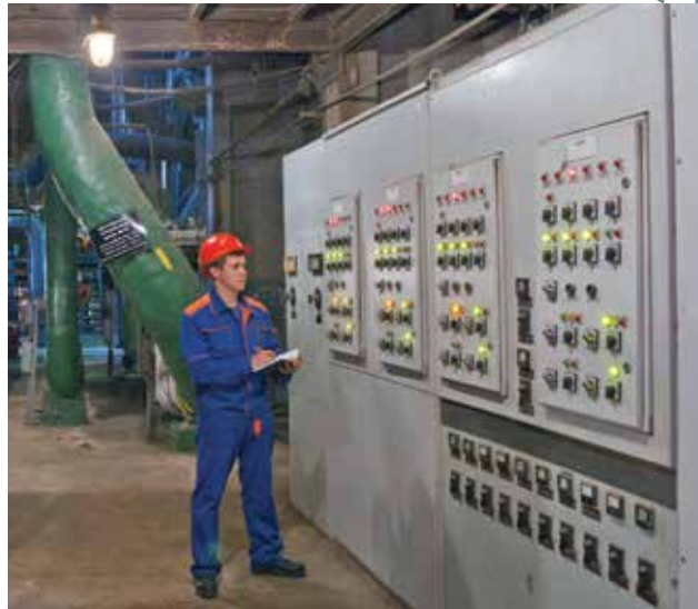
Local control switchboard for Boiler Unit #10
