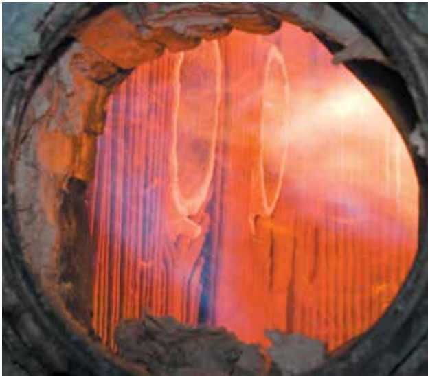
Boiler Unit furnace. Heat is made here
