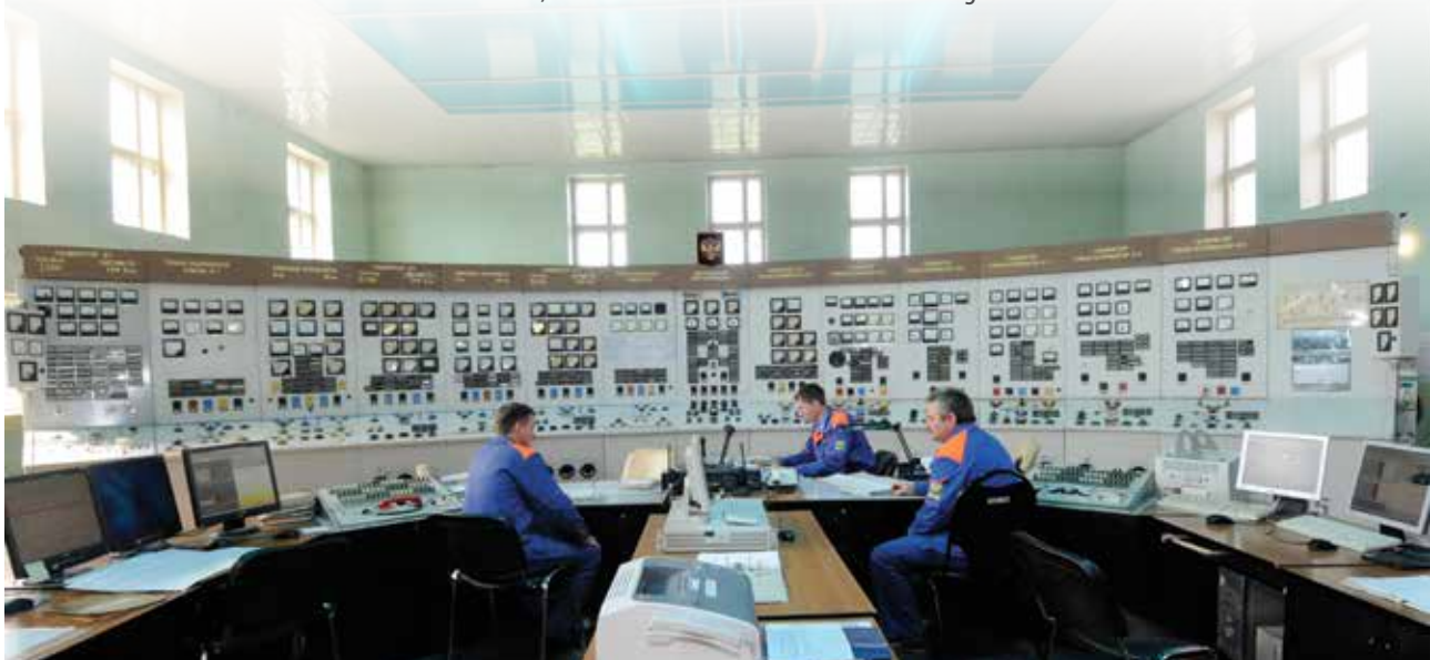
CHP Plant's main control board
