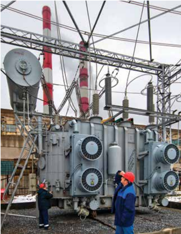
Power Transformer #5T
