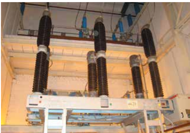
SF6 circuit breakers of additional 110 kV closed switchgear bays
