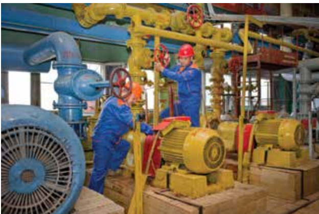
Pump facility of Chemistry Department's CWT-2
