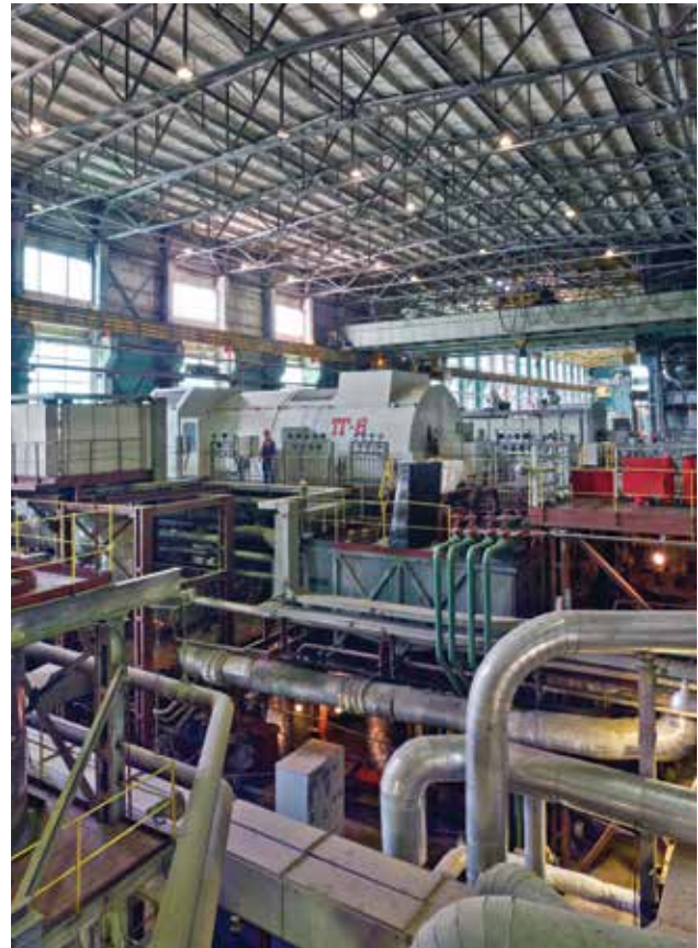
Turbine Department. Cogeneration Turbine #6
