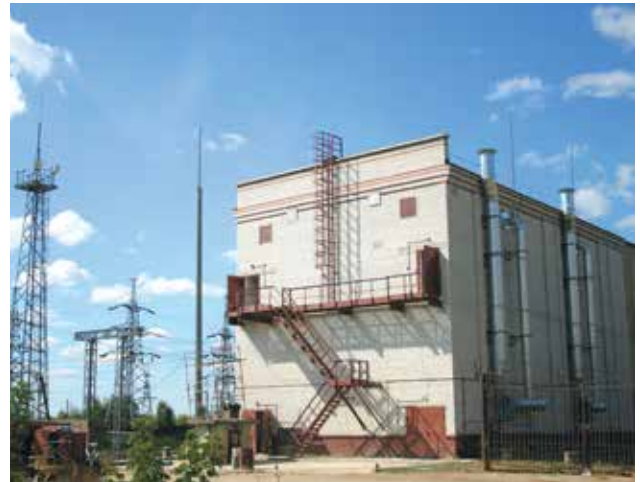
110 kV closed switchgear bays
