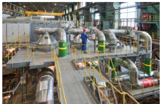
Delivery water pre-heating plant
