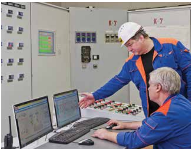
On the control switchboard for Boiler Unit #6
