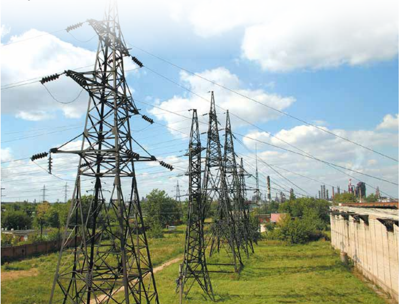
Power lines from CHP Plant to industrial consumers
