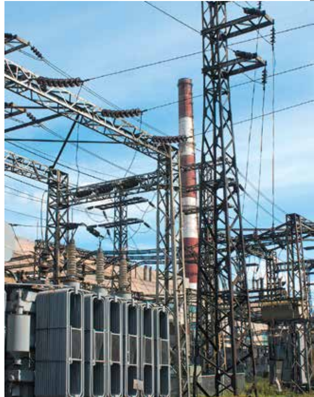
Exposed part of switchgear
