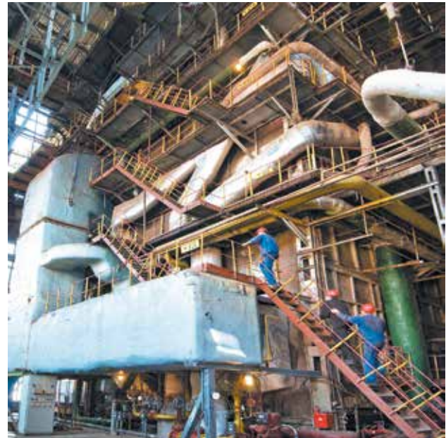
Boiler Department. Boiler Unit #1
