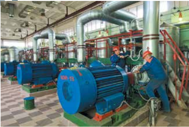
New fuel oil facility's pumps
